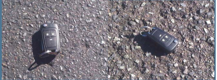
Condition of asphalt surface of local roads in Wallsend, Newcastle Council Left photo, Claymore Close - surfaced in 1992 and treated with Aspen Right photo, Boambee Close - surfaced in 1995 and no treatments to date
